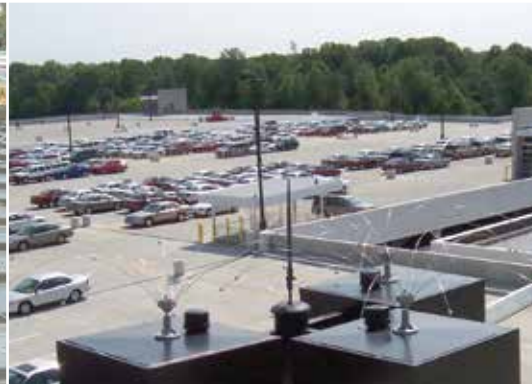
Three Daddi Long Legs protect these box lights on a large parking structure.
