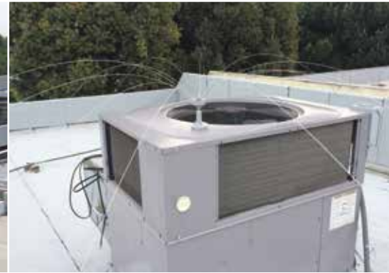
An eight foot Daddi Long Legs with magnetic base protects this large HVAC unit.
